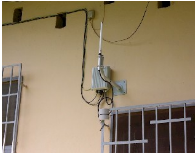
Fig. 16: Victoria Center Omnidirectional Access Point
