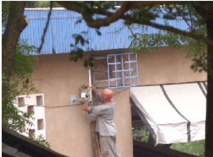
Fig. 13 – The omni directional Access Point in the Psychiatry building
