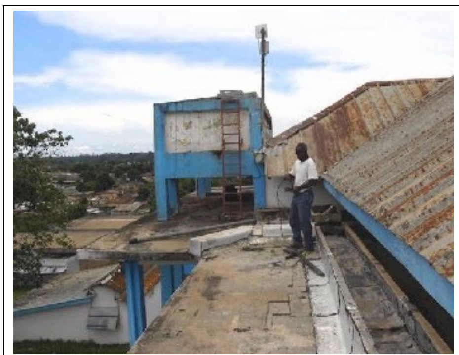
Fig. 9 – The Wifi antenna in the CHR Chateau d'Eaux
