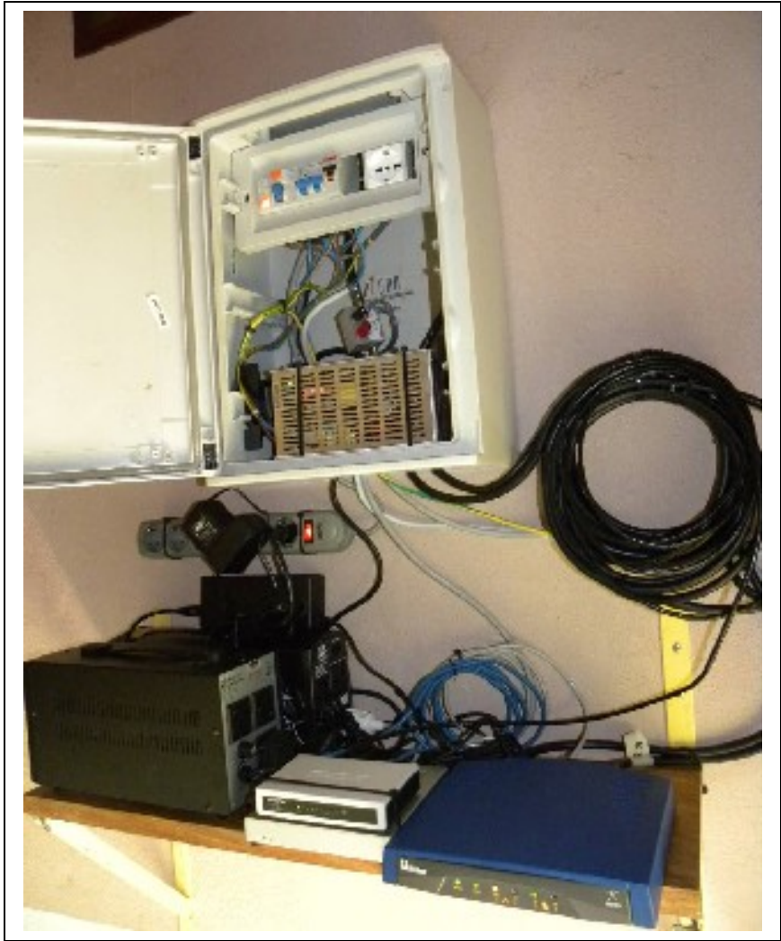
Fig. 5 – The IDU, Bias Tee, Power Supply and the rMain router
